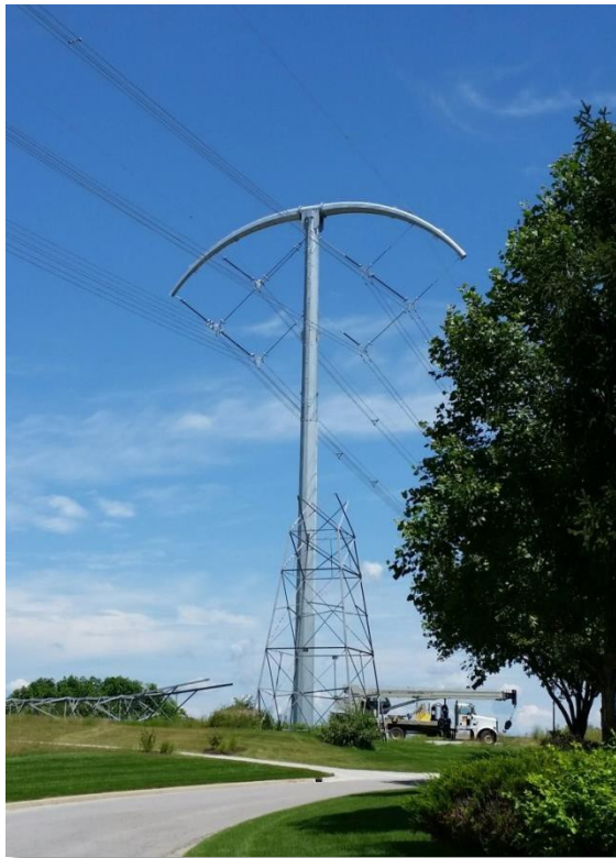
Figure 1: BOLD installation near Fort Wayne, Indiana
